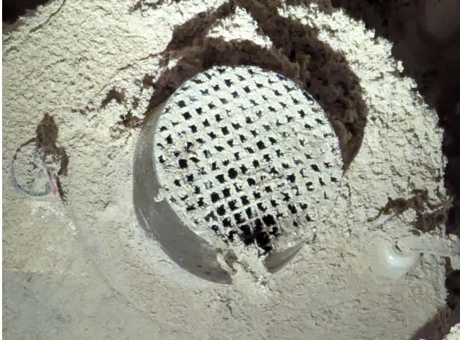
Figure 4. The air intake screen on this tube heater was clogged with caked dust and moisture.
