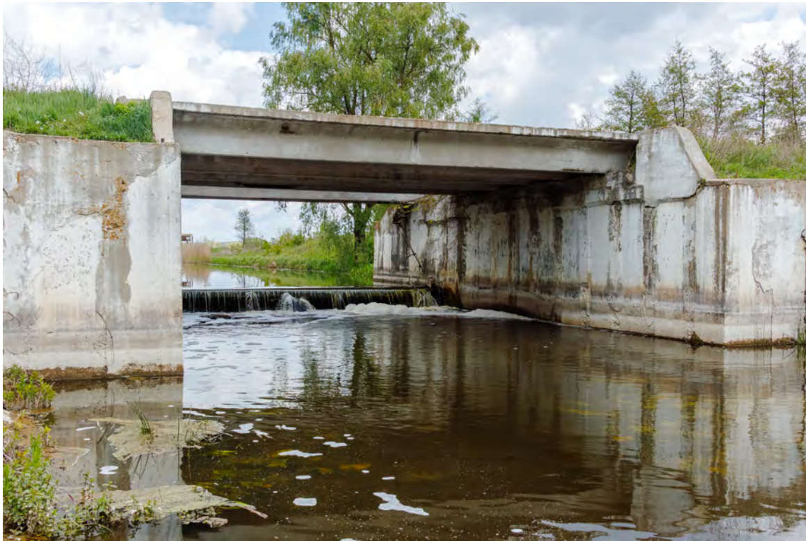
Figure 34. Stream barriers alter the natural flow of the water body and can pose hazards to human safety and the aquatic environment.
