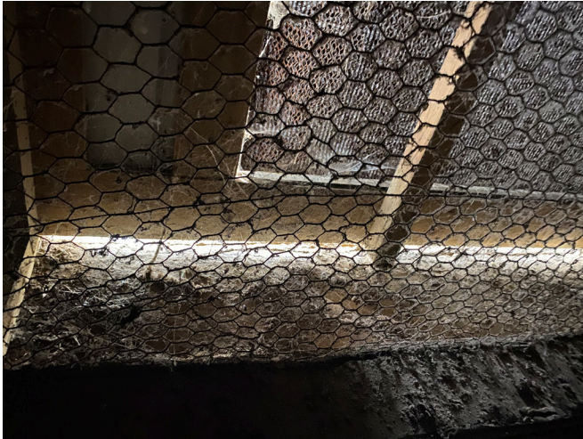
Figure 2. Can you identify the problem or problems in this picture taken from the inside of a broiler house looking through the tunnel inlet? A. Cobwebs on pads, B. Cobwebs on bird wire of inlet, C. Light and air leak entering between the floor and wall of the doghouse, D. Floor is dirty, E. All the above. If you answered E. (All the above), you would be correct. This doghouse and pad system are not ready for hot weather.
