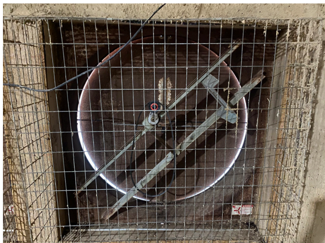
Figure 1. Can you identify the problem with the fan in this picture? A. No motor, B. No propeller, C. Not clean, D. All the above. If you answered, D (All the above), you would be correct. Also note that the adjacent tunnel fan #3 is plugged into the outlet above this fan, tunnel fan #1. This fan is not ready for hot weather.
