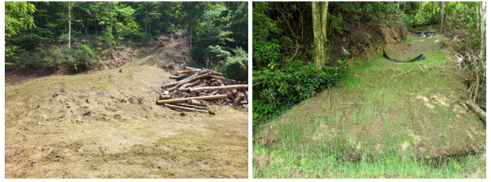
Figure 11. Grass seed and straw (left) and grass seed and silt fence (right) implemented as a close-out BMP on skid trails to stabilize the soil. Silt fences help slow down runoff and erosion that, in turn, can help grass seed germination. (Photo credit: (left) Andrew Vinson, Virginia Department of Forestry and (right) North Carolina Forest Service)
