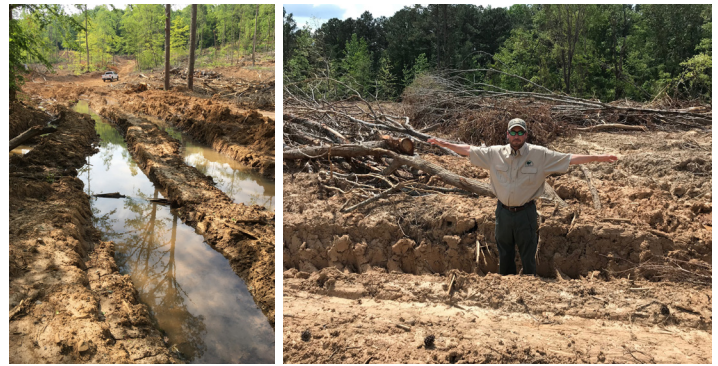
Figure 3. Excessive rutting caused by a skidder. These types of ruts need to be avoided, and if they do occur, they should be fixed before leaving the site. Avoid deep rutting by waiting to harvest a tract or section of the tract when there has been significant rainfall (harvest during dry time of the year) or implement BMPs, such as placing logging slash or wood mats on the skid trail to skid over.
