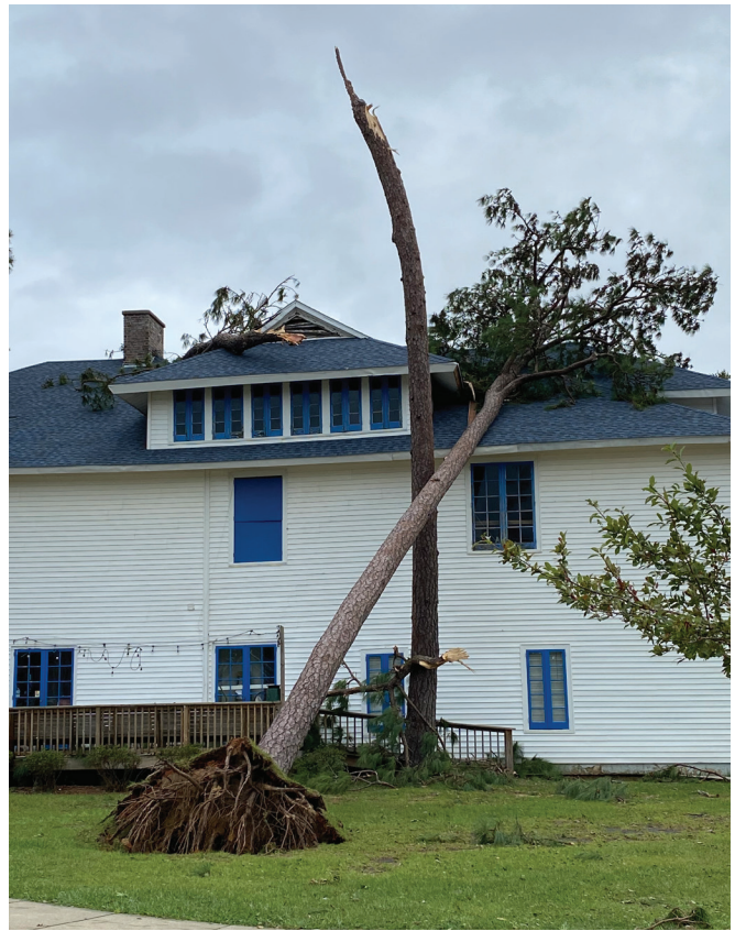
Figure 16. Large trees on structures often require large equipment to safely remove them.
