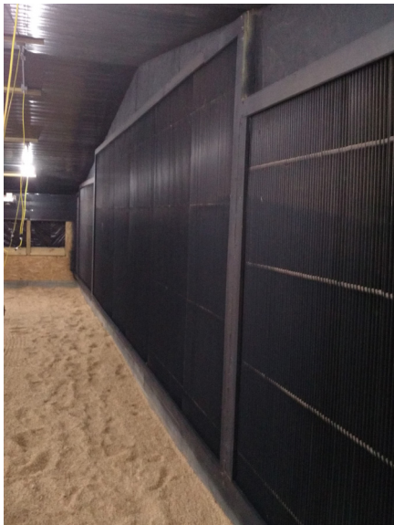
Example of a dark-out “false-wall.” Behind this wall, unseen to the right, are exhaust fans pulling air through it to ventilate the house. The false wall keeps light from entering the house when the fans are operating. Similar components are on every air inlet and exhaust fan in a dark-out pullet house and all must be kept clean and maintained.
