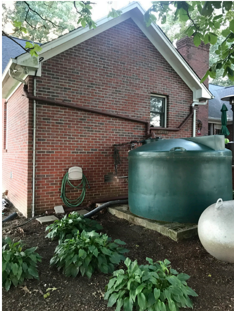
Figure 13. Rainwater harvesting tank with downspouts and first flush diverter
