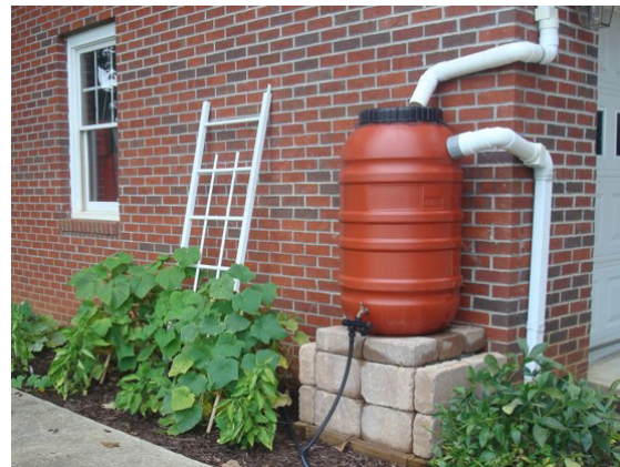
Figure 29. Elevated olive barrel collecting rooftop rainwater with overflow valve directed to downspout; hose connected for watering nearby plants
