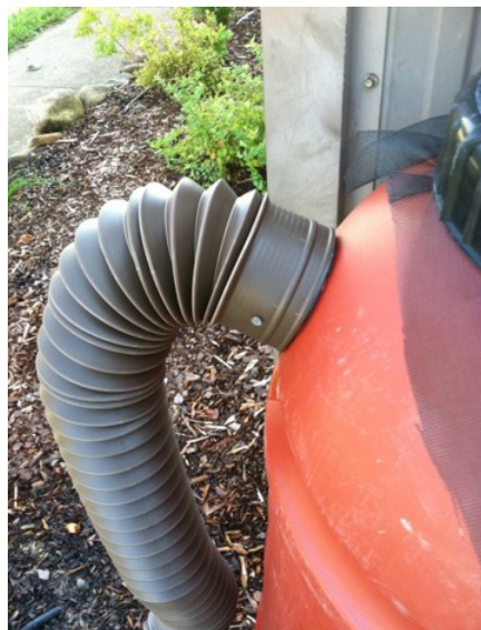
Figure 22. Olive barrel with overflow pipe to divert excess overflow away from foundation
