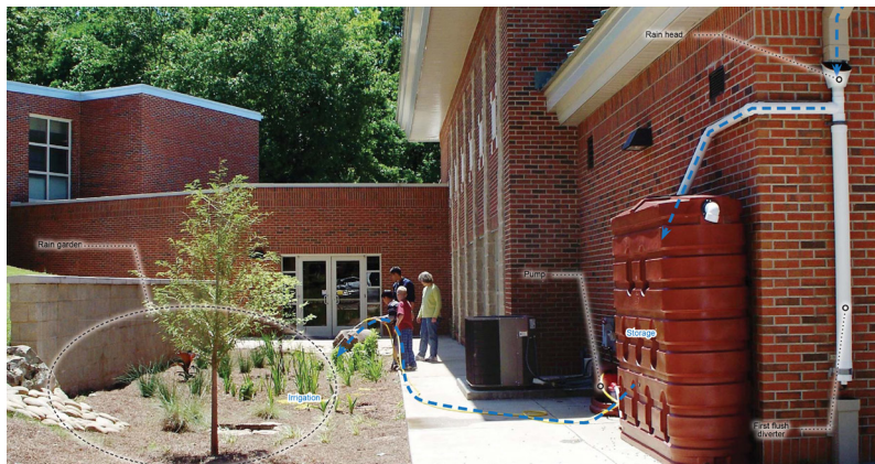
Figure 14. Cistern in use with a rain garden. Note the prefiltration devices on the right including the first flush diverter and rain head collecting water from the downspout.
