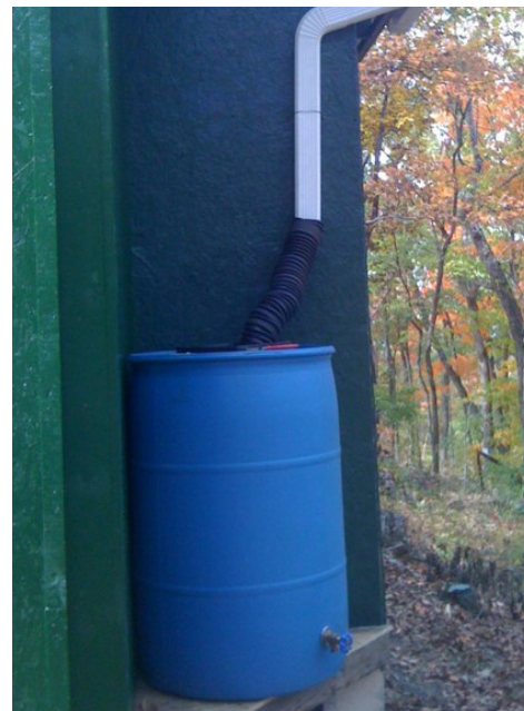
Figure 28. Repurposed soda/syrup barrel collecting roof water. These barrels are sealed at the top and are typically blue or white.
