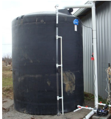
Figure 11. A 3,000-gallon rain cistern, Moulton, Alabama
