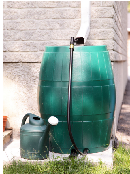
Figure 18. Gutter and downspout directing water to ground. This would be a potential area to intercept water from a downspout and transfer it to a rain barrel or cistern.
