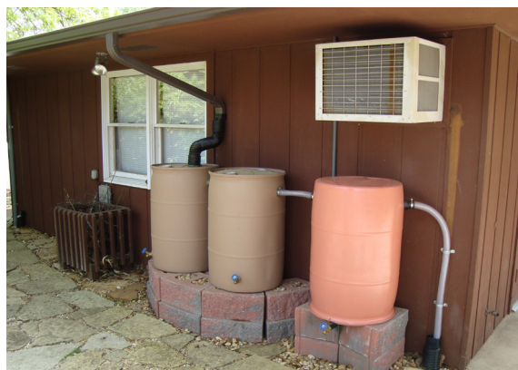
Figure 36. Rain barrels collecting water with gutter diverter, with linked connected overflow eventually directing excess into downspout
