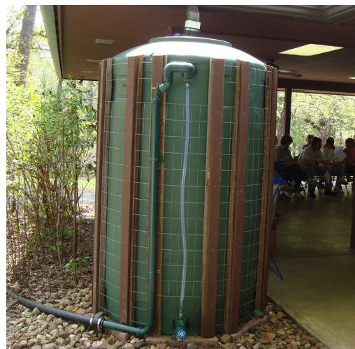
Figure 12. Cistern collecting rooftop rainwater through gutter system
