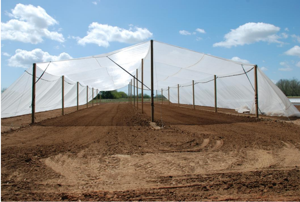
Fig. 1. Semi-completed structure of net house (50-mesh fabric) showing poles and sloping side walls. The center poles are 17 ft tall and the side poles are 14 ft tall. Location: Allegri Farm, Fairhope, AL.
