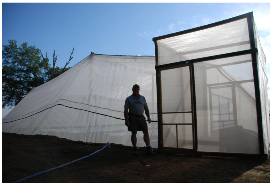
Fig. 4. Construction of the double door and sealing of the net house. Vince Allegri (in picture) of Baldwin County became the first user of a net house for vegetable production in Alabama.
