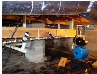
Pump, pipes, and water flow control in the crawl space
