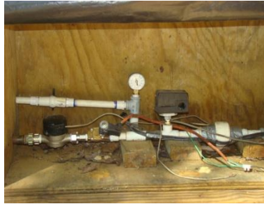
Flow control in the crawl space
