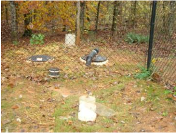
Underground storage tank with buried pipes
