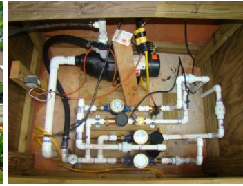
Pump and water flow control in an insulated wooden box
