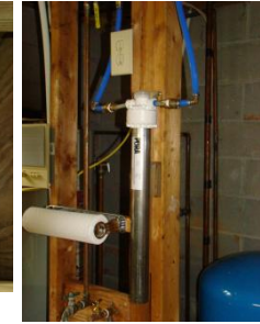
UV tube in the basement
