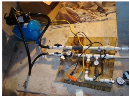
Water flow control, pump and pressure tank located in the basement
