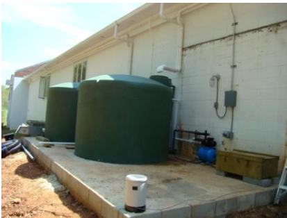
Storage tanks and roof lines before an insulated shed was built to house the RCR
