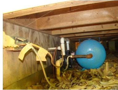
Pump and pressure tank located in the crawl space
