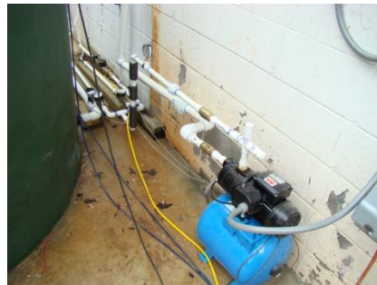
Pump and pressure tank
