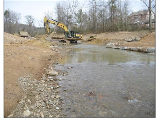
In-stream structures direct flows away from the streambanks to the center of the channel.
