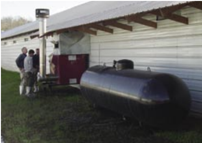
Specially designed waste-oil furnaces installed on five Alabama farms have enabled growers to reap huge savings in energy costs.
