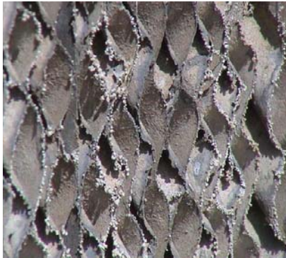
Scale accumulating on the edge of pads.
