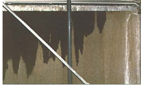
A water distribution pattern on a pad showing less water along the pad length from a clogged distribution head.
