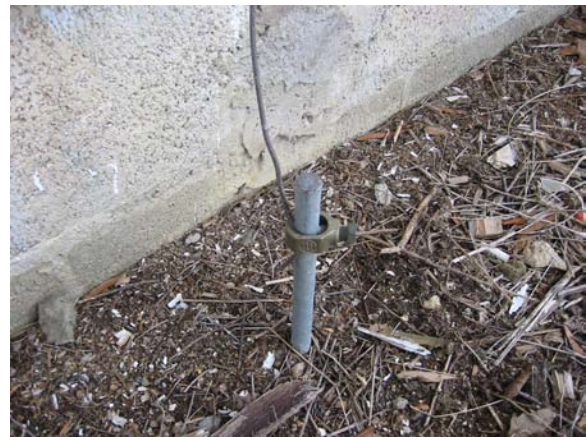
A typical ground rod, acorn clamp and ground wire installed above grade close to a house wall.
