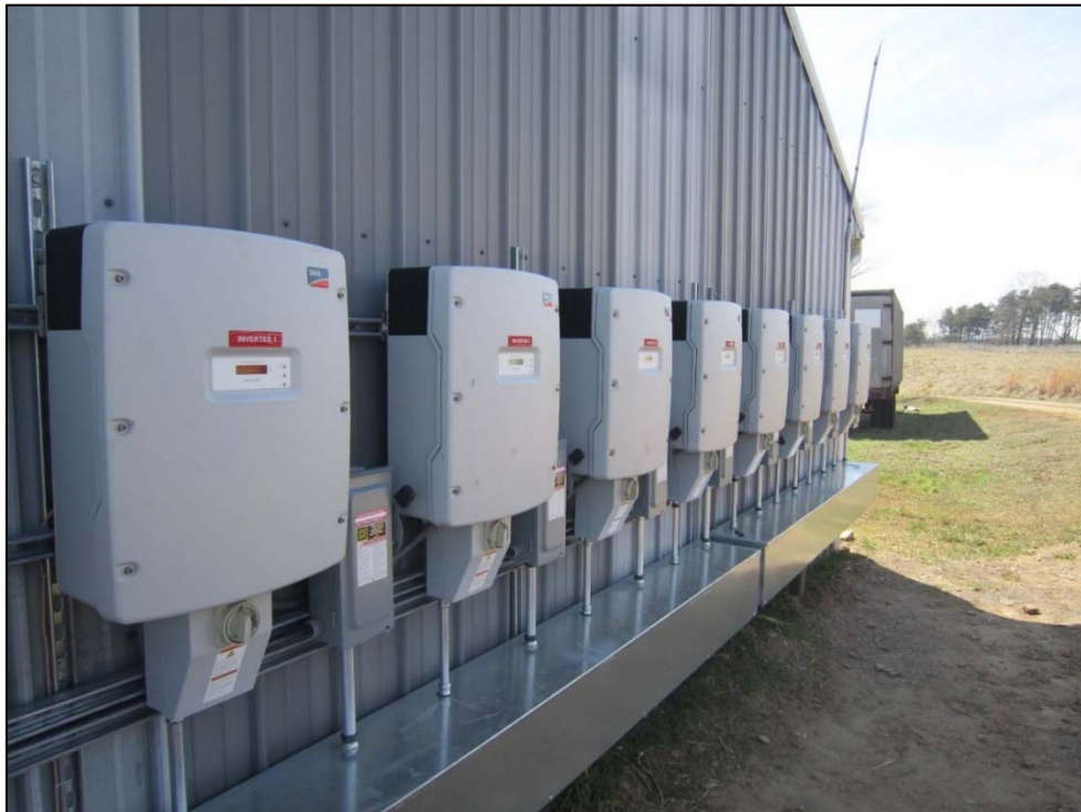
Figure 2: Solar systems use power inverters like the ones seen here to convert solar generated DC power to AC power capable of being fed back onto the utility company power grid.
