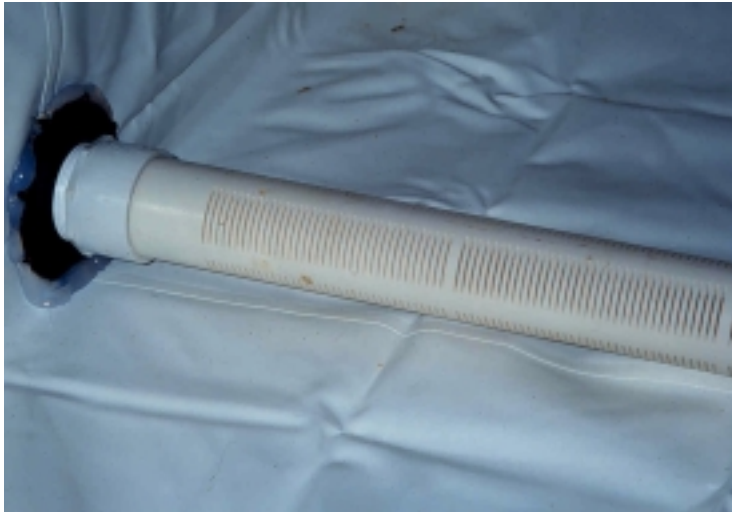
Picture 1 Illustration of the 20 mil plastic bed liner and bulk head fitting and well screen - drain.
