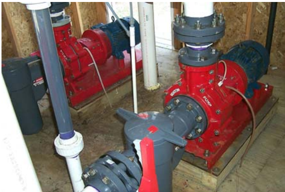
Figure 6. Dual intake pumping system.
