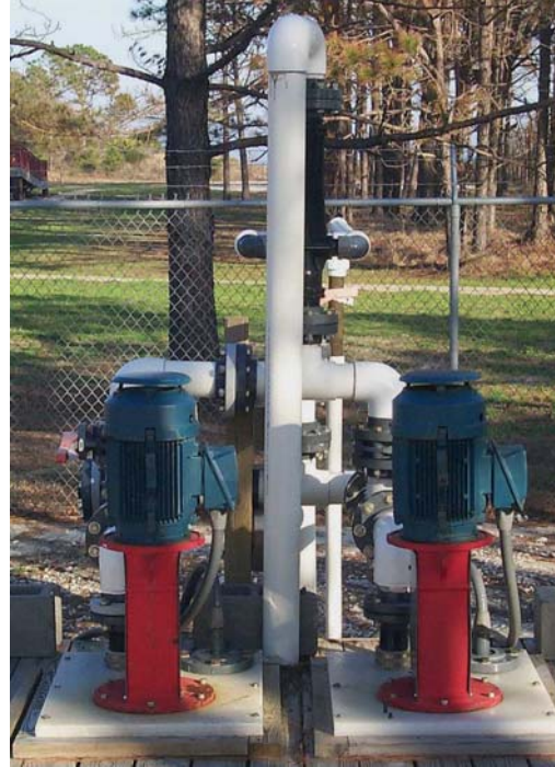
Figure 7. Dual discharge pumping system.
